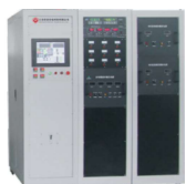
Control System: Human Machine Interface (HMI)
